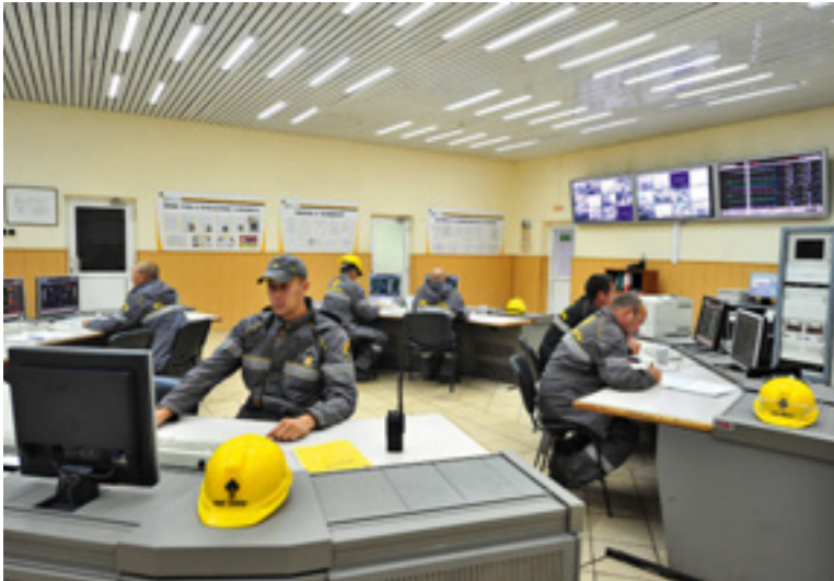
36 page ▲ Control room of primary oil treatment plant at the Syzran Refinery
