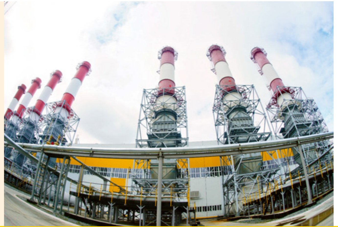
▲ Gas turbine plant at the Priobsk field
